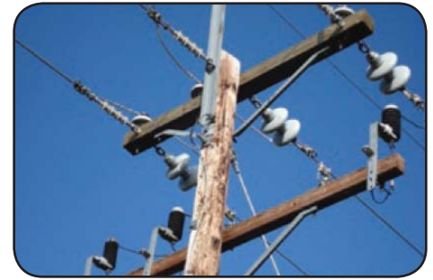
Power lines before the bird proofing project.
